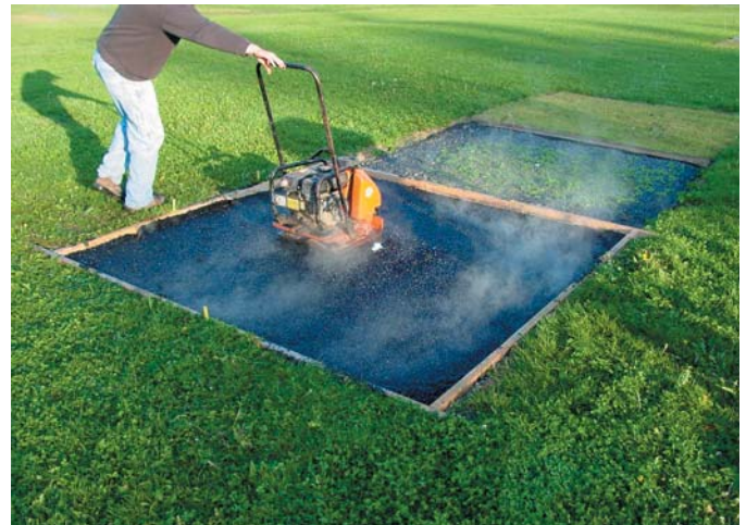
Fig.1.14 Compaction of porous asphalt on CU-Structural Soil® in a test plot on the Cornell University campus.
