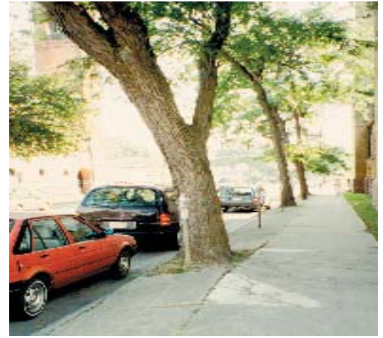
Fig. 1.20 Sidewalk heaving caused by superficial tree root growth, Ithaca, NY
