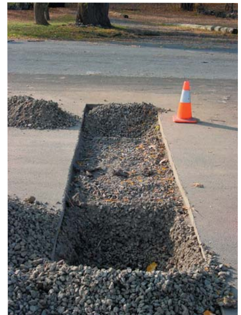
Fig. 1.24 In this parking lot, there is only a 3 foot opening for tree planting. Here CU-Structural Soil® was installed underneath the asphalt to extend the rooting volume for the trees. Once the pavement was cut, bare root Accolade Elms were planted in November 2005.
